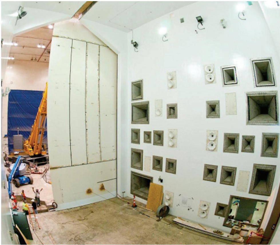
Figure 2: Ongoing Construction of the NASA Reverberant Acoustic Test Facility (RATF). The modulators are located behind the horn wall shown in the photograph.
